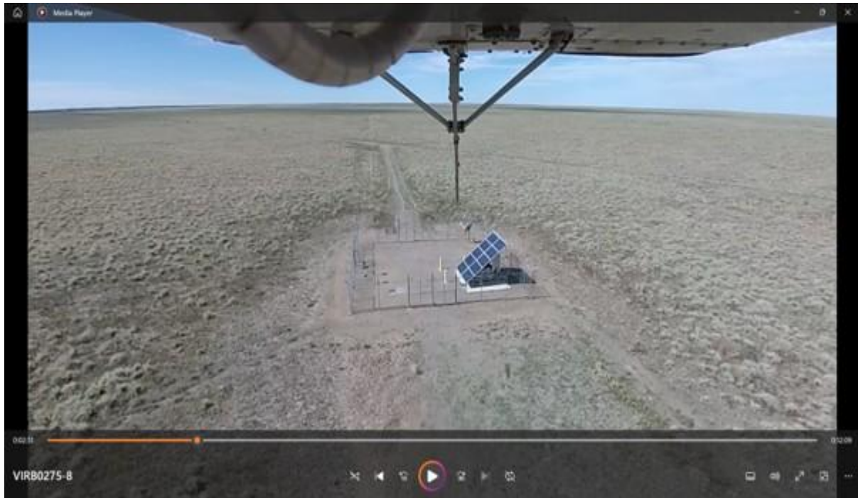
Photo: Cathodic protector – no weeds inside of infrastructure (2.51s)
